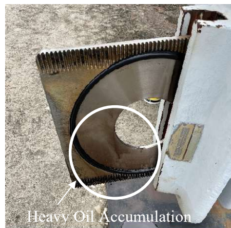
Figure 1. Orifice Plate Contaminated with Oil
